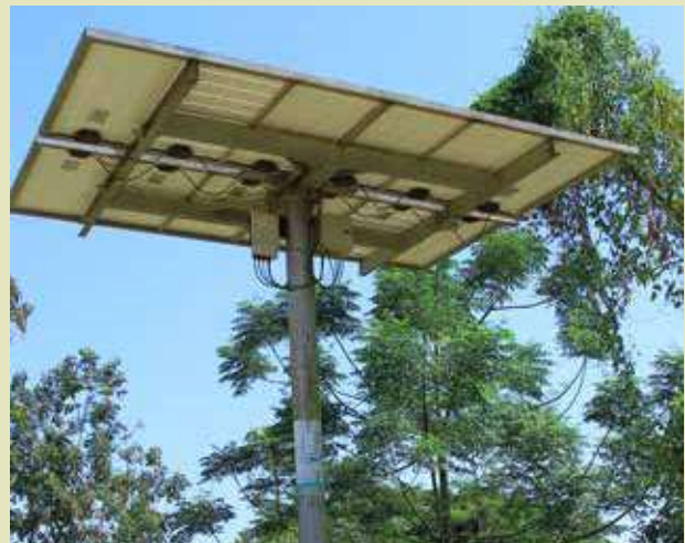
Solar powered water pump panel
